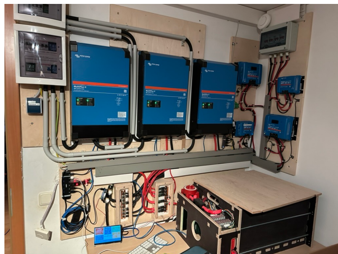
v1 of SAFEr Grid capability: grid forming PV with battery
